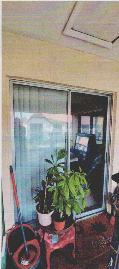
Unprotected glazed entry door
