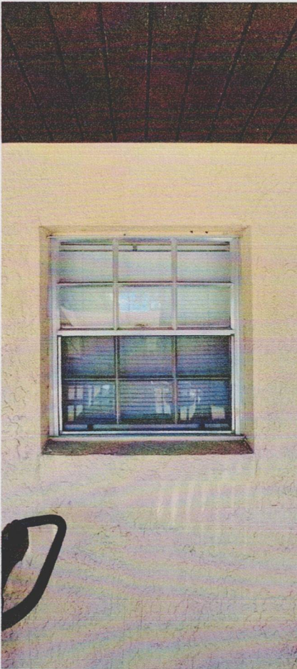
Unprotected glazed opening
